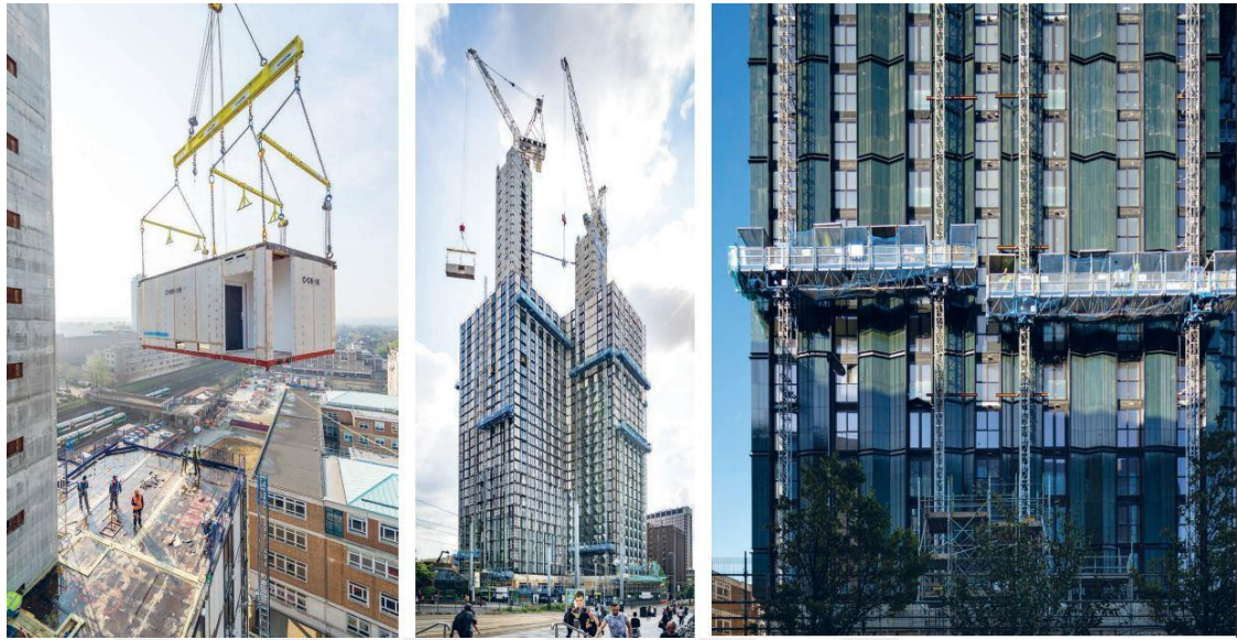
Figure 4.3.9 The construction process of Ten Degrees, craning, installation of modules, and façade works (Bayliss & Rory, 2020)
